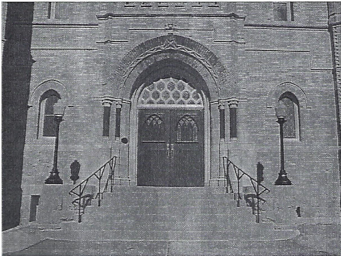
Main east entry - double doors, brick arch indentation detail, stone detailing, stone base, columns, foundation light supports
