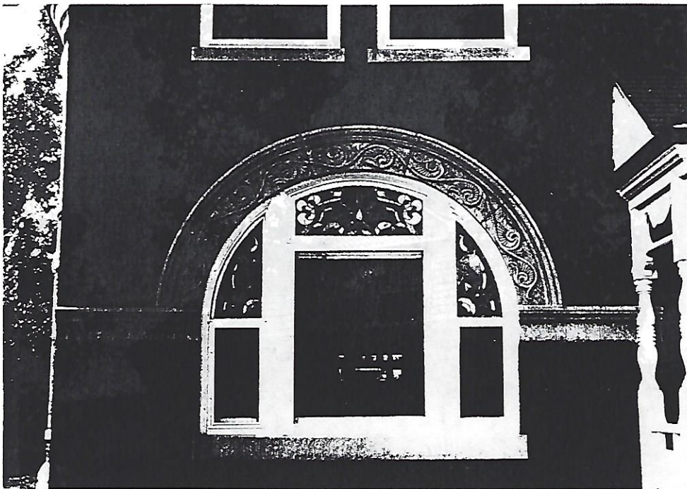
Detail of the semi-circular arch window on the North facade with carved stone arch, stone sill, carved wood frame, stained glass toplight and stone beltcourse extending from the sides
