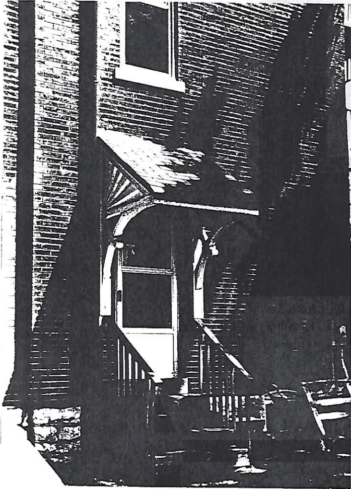
South facade entry with wood frame hood that has brackets and carving, and stone threshold
