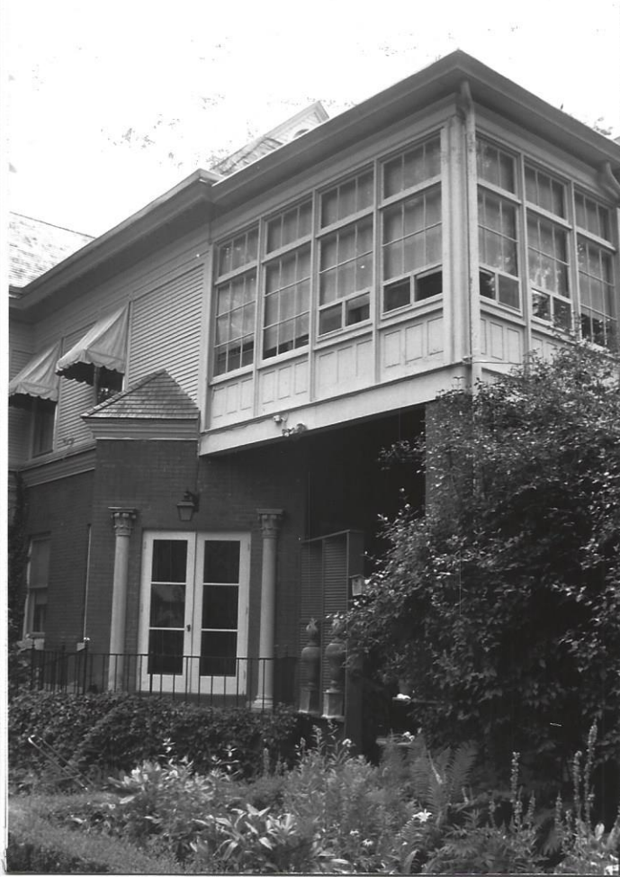
Detail of the sleeping porch on the second story of the rear wing with wood frame, windows and supported by a brick pier
