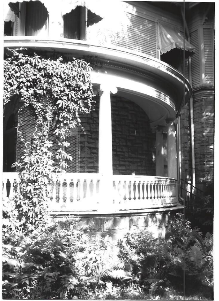
Detail of the Southeast corner of the wrap-around porch with Ionic columns, wood vaulted ceiling, wood railing and turned wood balustrade, and wood cornice with dentils
