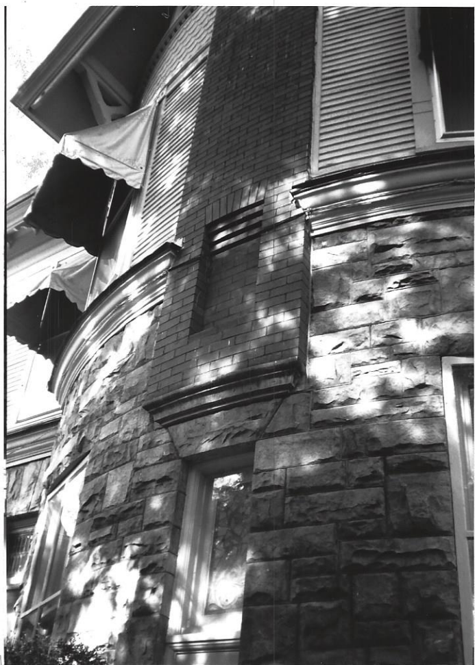
Detail of the lower part of the East chimney, also shows the stone first story and the wood siding on the second floor
