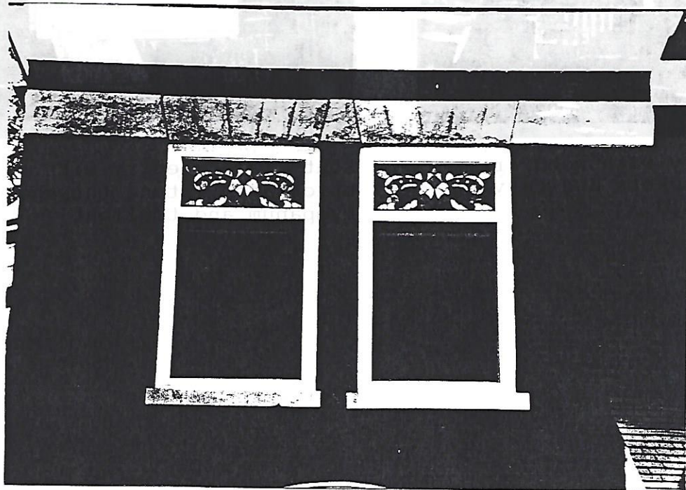
Second story windows on the North facade with stone lintels and sills and stained glass toplight
