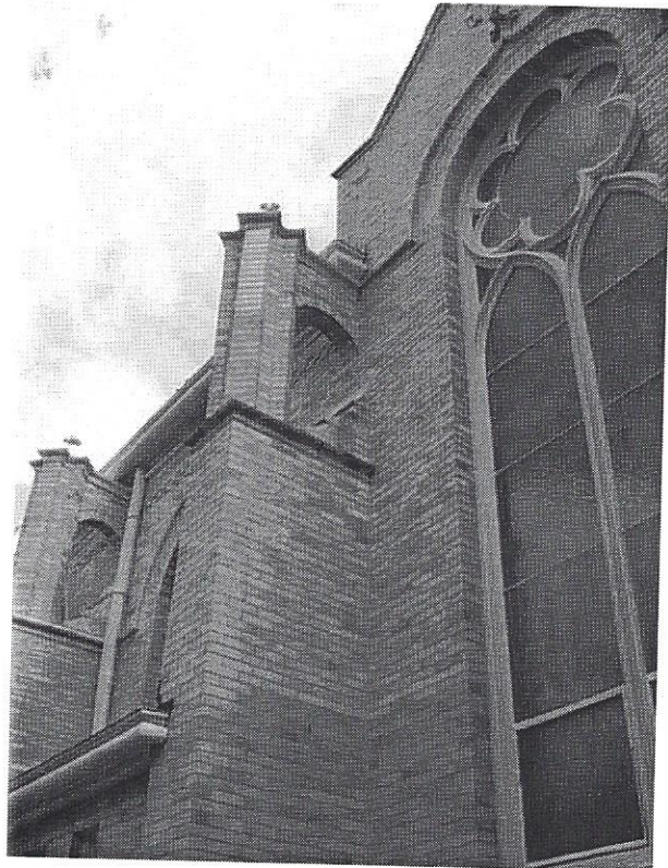
“Buttress arch column” - engaged brick column with decorative column on top, stone buttress detail, brick arch, finial (north side picture)
